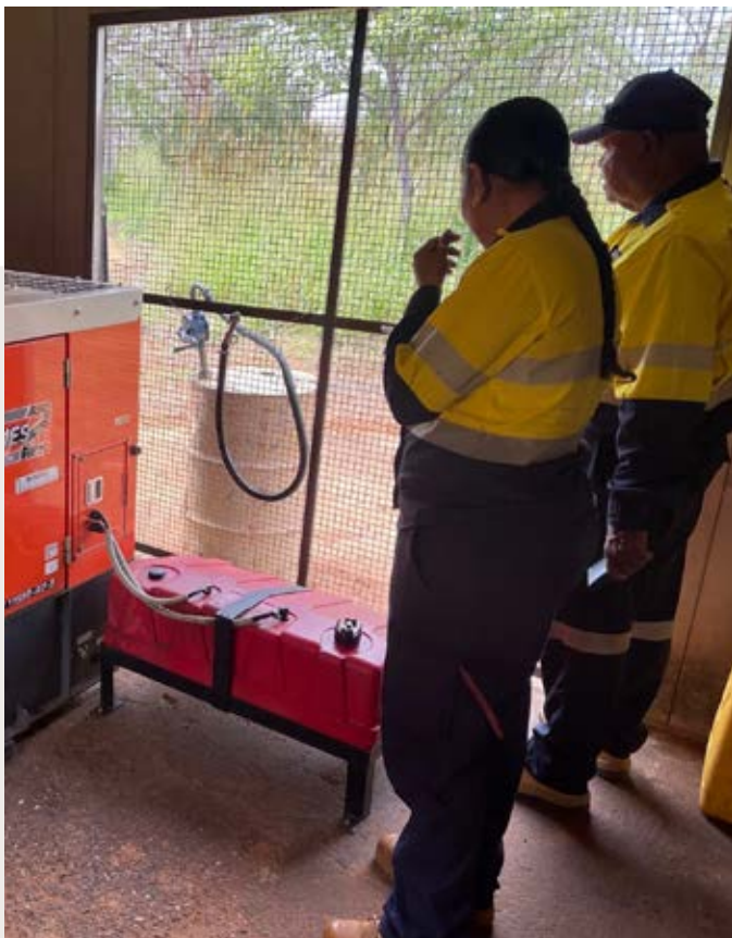
Terry Shadforth and Apprentice Power Worker Simone Long inspect existing power assets in a remote community
