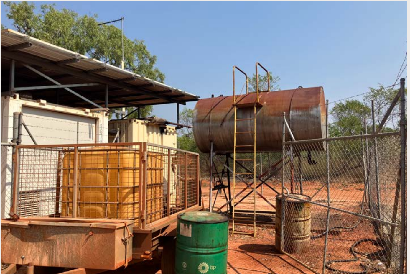
Power assets in a remote community
